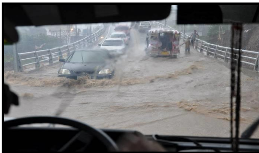
Figure 25. Flooded Flyover in Cagayan de Oro
